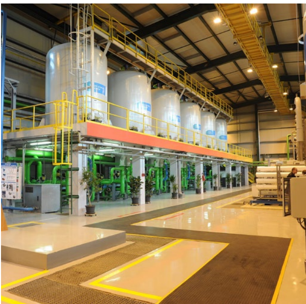
The water in the technological process is constantly purified and reused
